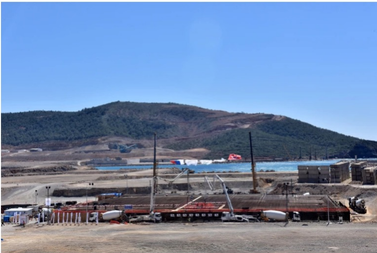
A view of the construction site of Turkey's first nuclear power plant 'Akkuyu', pictured during the opening ceremony in the Mediterranean Mersin region on April 3, 2018 [File: Ibrahim Mese/AFP]
